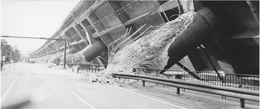
Gambar 1. 1. keruntuhan Higashi-Nada Viaduct (Rute 3) (Duan & Chen, 2003)
