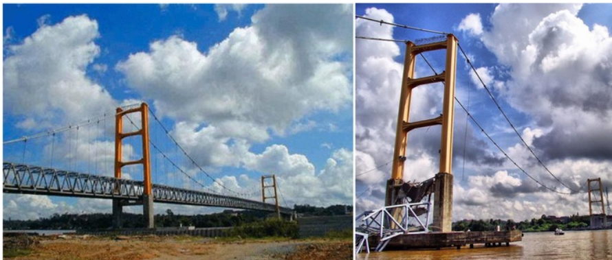
Figure 2. Kutai Kartanegara Bridge before and after collapse [7]
